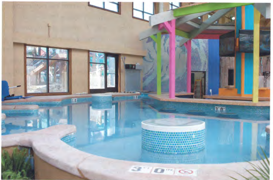
As crews put the finishing touches on the swim-up bar, extensive plan modifications beforehand made construction possible. Beginning plans rarely matched as-built portions already in place, so the design build team made, reviewed and approved changes practically on the go.
