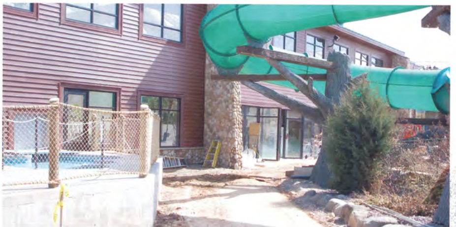
Inside the courtyard, this was the only path for equipment and supply traffic. The overhead support for the water slide created clearance issues. The base of the building buttress (center) uses salvaged face stone from other parts of the building for a good match.
