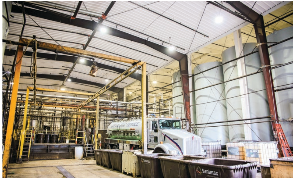
The interior of the structure illustrates the complexity of this facility with its extensive plumbing and tank storage. Work was completed in phases to allow for minimal disruption of operations.
