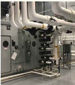
Exact Sciences Mfg. and Clinical Science Building / North American Mechanical, Inc. (HVAC)
