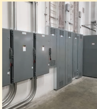
MGS Clean Room Steiner Electric, Inc.
