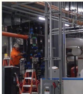
Exact Sciences Mfg. and Clinical Science Building / North American Mechanical, Inc. (HVAC)
