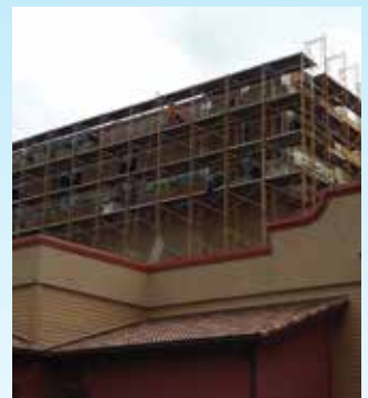
Chula Vista Resort Fire Restoration / Friede & Associates
