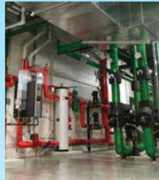
Great Lakes Energy Education Center, Northeast Wisconsin Technical College / Performance Firestop, Inc.
