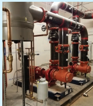
The James, North American Mechanical, Inc.
