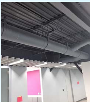
QBE Building 300, North American Mechanical, Inc.
